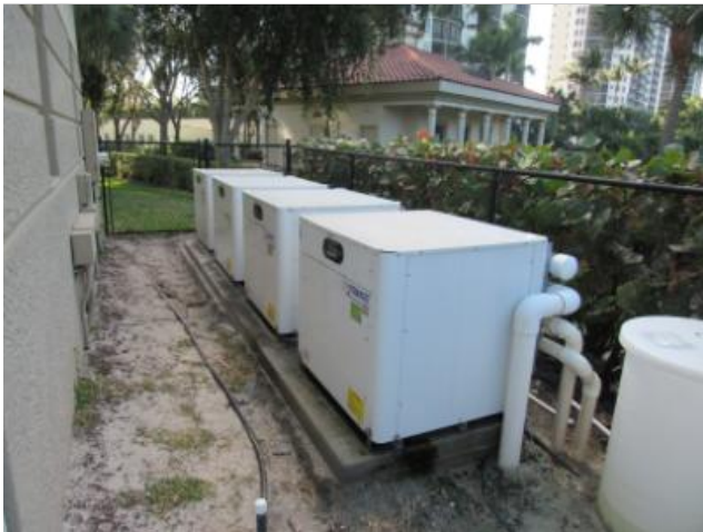
View of subject geothermal pool heaters.
