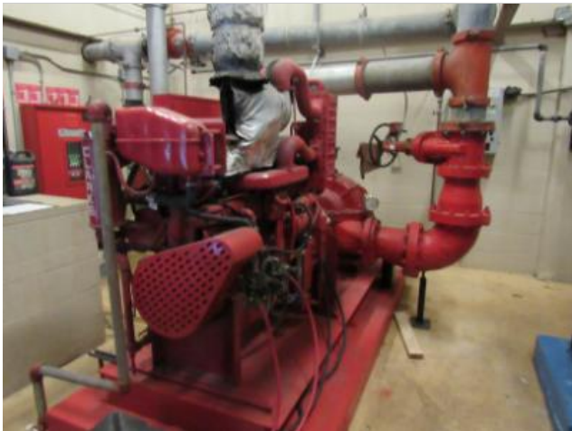
Typical Fire Pump and related equipment observed during our site inspection.
