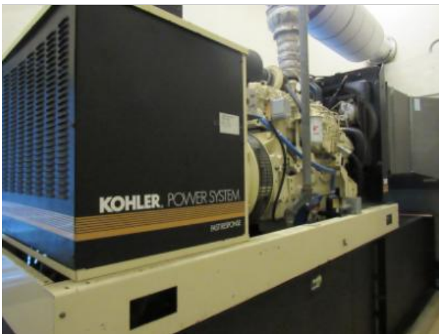
200 kW generator observed during our site inspection.
