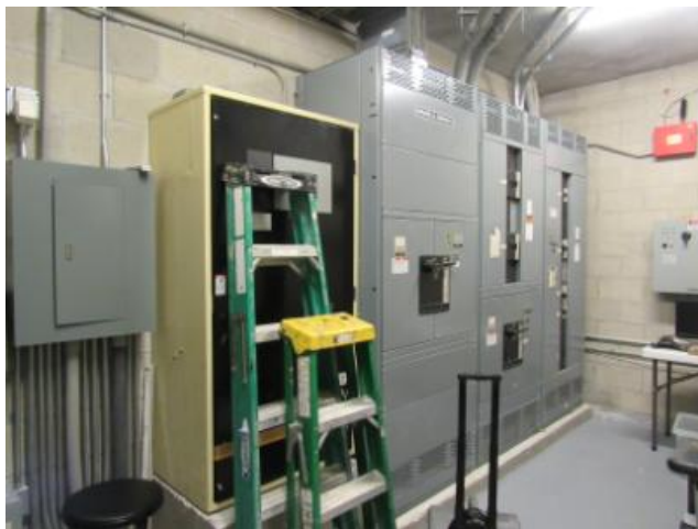
Typical electrical system components observed during our site inspection.
