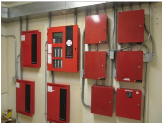
Typical Fire Alarm System components observed during our site inspection.
