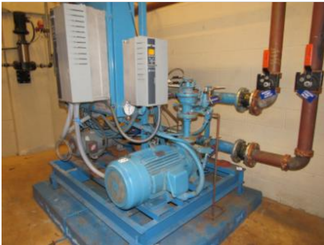
Typical Domestic Water Pump and related equipment observed during our site inspection.
